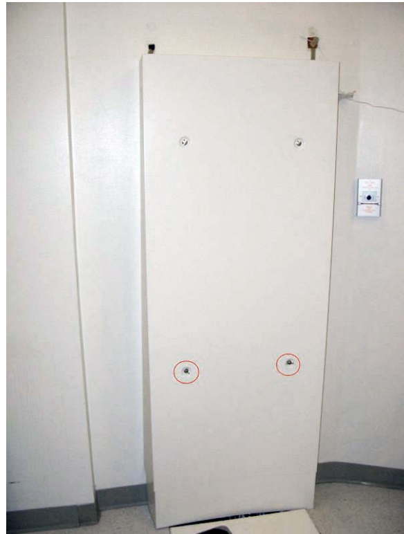
Two of four shield panel fasteners were found missing in the MRI room (red circles).
