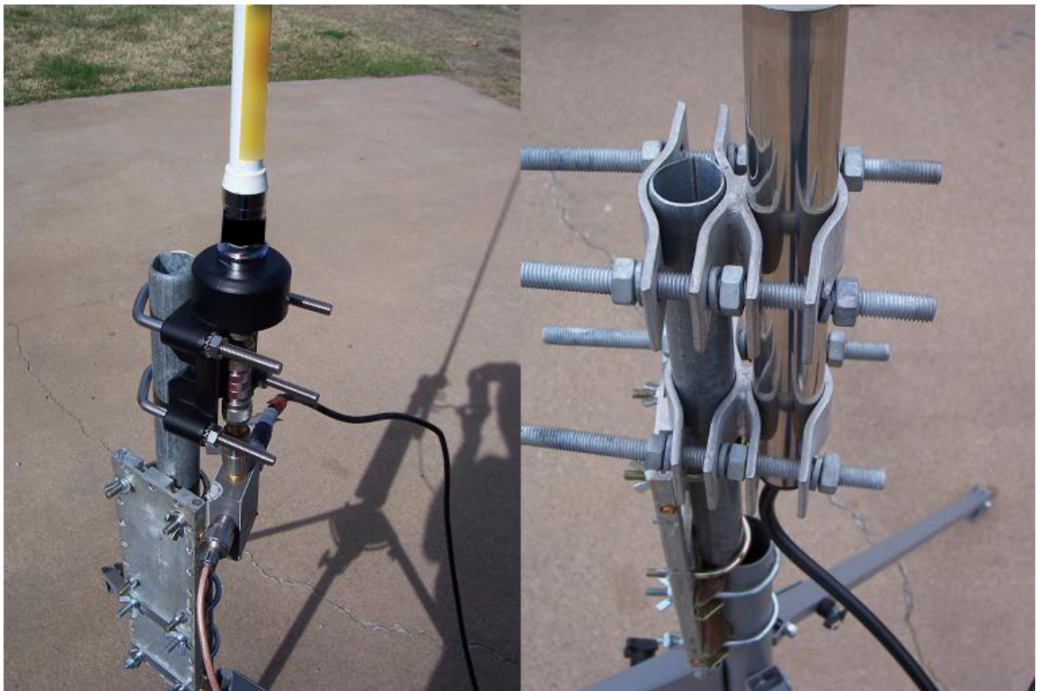
Above Left: Base of Brand #3 antenna. Right: Brand #1 antenna base clamps. Note the VSWR directional bridge connected to the Brand #3 antenna.
